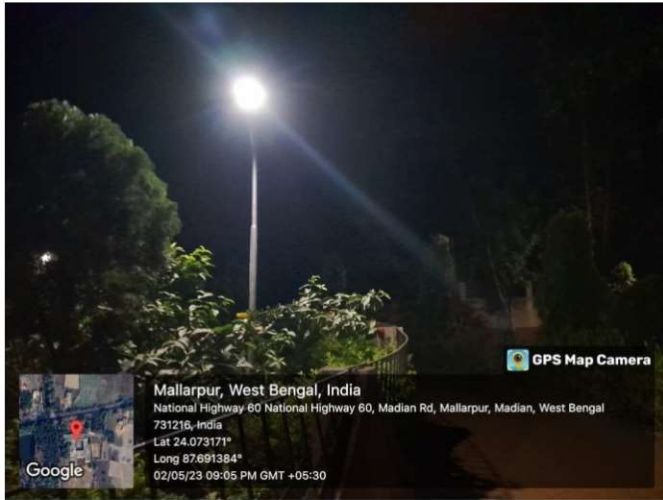
Figure 1a: The street light has been installed inside the Butterfly Garden situated in front of the institution.
