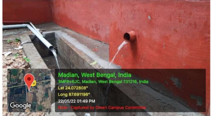
Fig2. Rain water comes from west side portion rooftop and central yard of the main campus.
