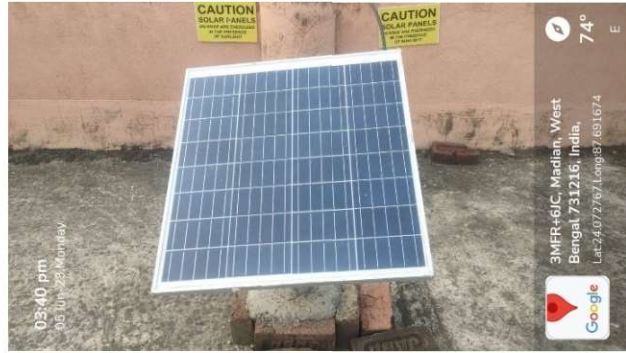
Figure 1e: The solar panel of figure 1c. The panel is fixed in the roof top to perceive sufficient sun light.
