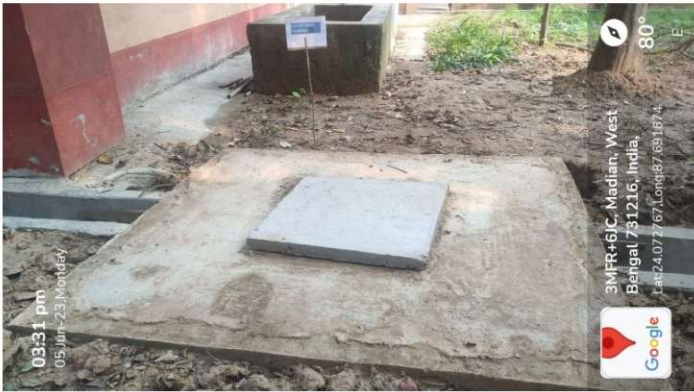
Fig 1: Ground water recharge chamber constructed in Medicinal garden area which is in west side of campus.
