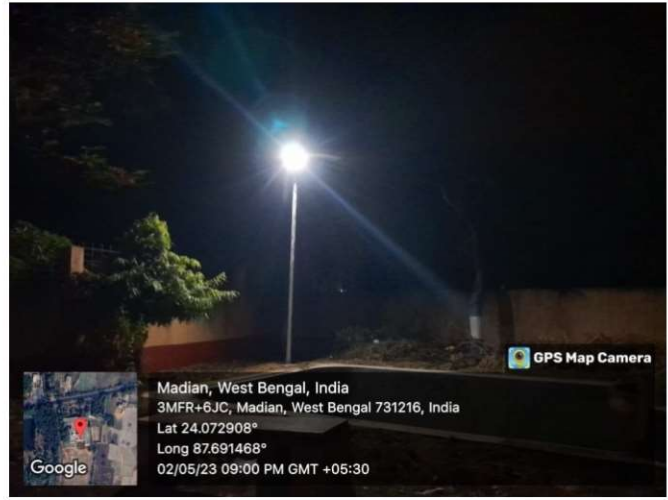
Figure 1b: The solar street light has been installed in East-North corner of the institute beside the rain water harvesting reservoir.
