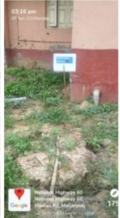
Fig 6: One of four soak pits for rooftop water and sewage of boys' toilet constructed in east side of the campus.
